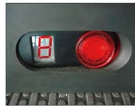
Fault Display for S and F Type
